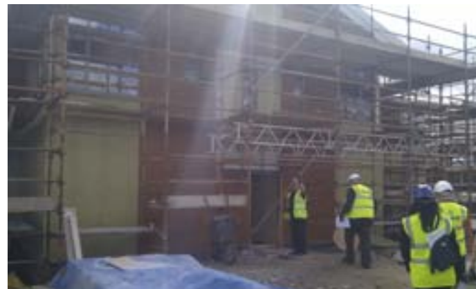
The front of the new child protection building in Dundee, near Kingscross hospital
